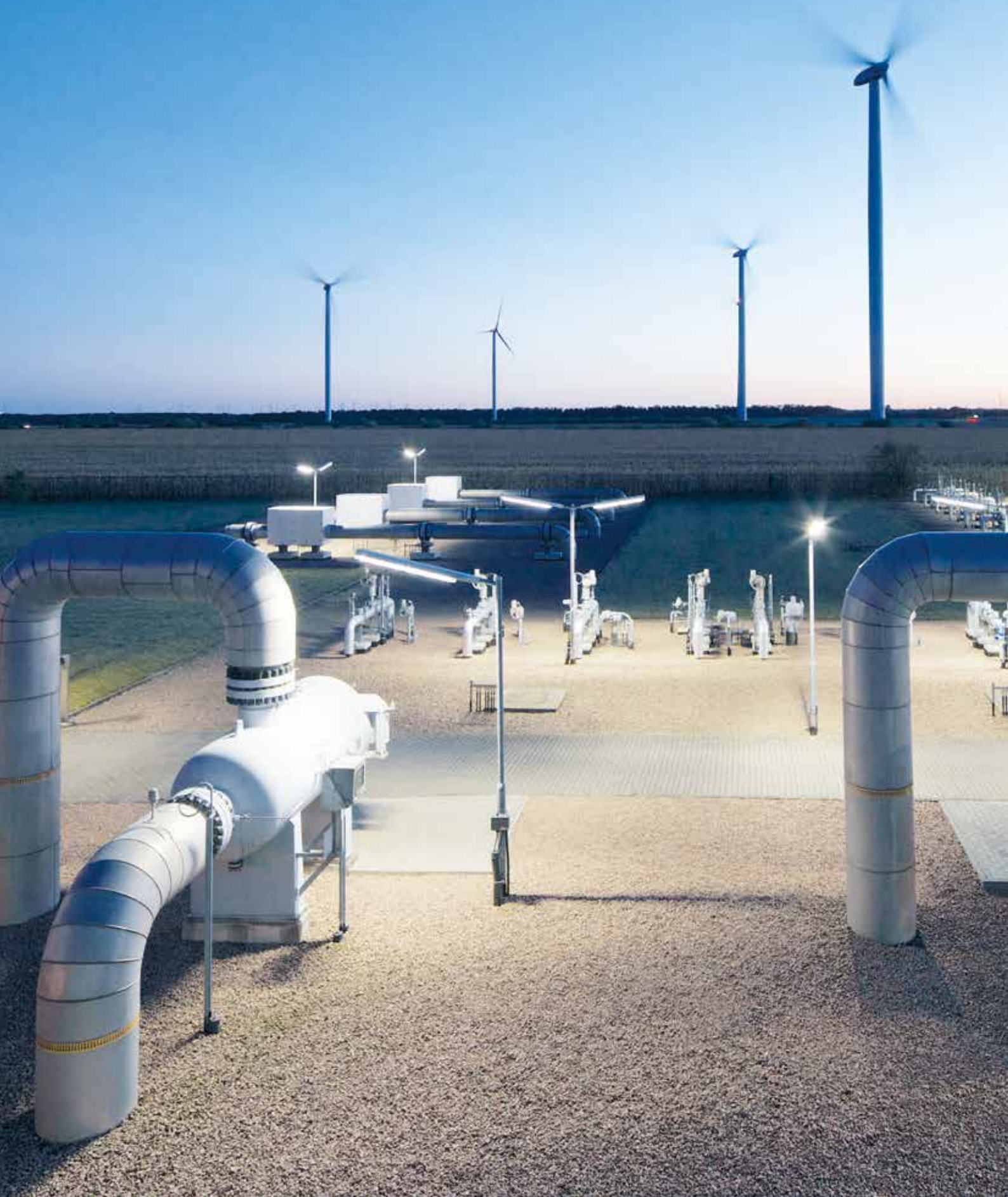
Gas control lines at a compressor station of ONTRAS in Bobbau (Saxony-Anhalt).
